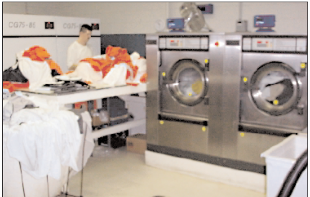
Sevier County's two 55-pound, soft-mount Continental Pro-Series™ washer-extractors and two 75-pound dryers have boosted the facility's production and slashed utilities.
